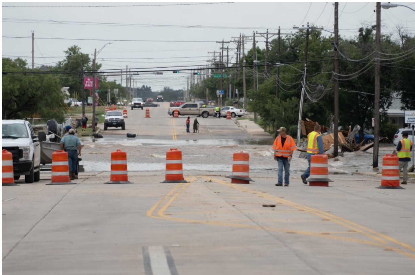
San Angelo flooding, damage, and recovery efforts. (Photos courtesy of San Angelo Emergency Management and San Angelo Police Department)
